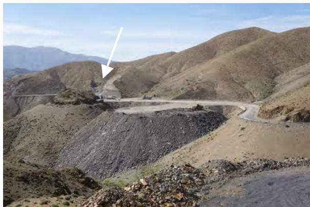
Fig. 92: Road construction site, new breakthrough with remarkable impact on the natural environment in progress (arrow). Area T1a, spring 2015.
