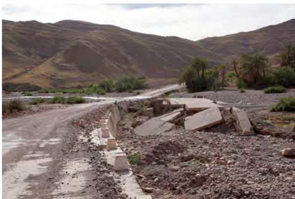
Fig. 224: Concrete ford destroyed by flooding of the Oued El Koubia. Domain C, area AS6d, spring 2015.
