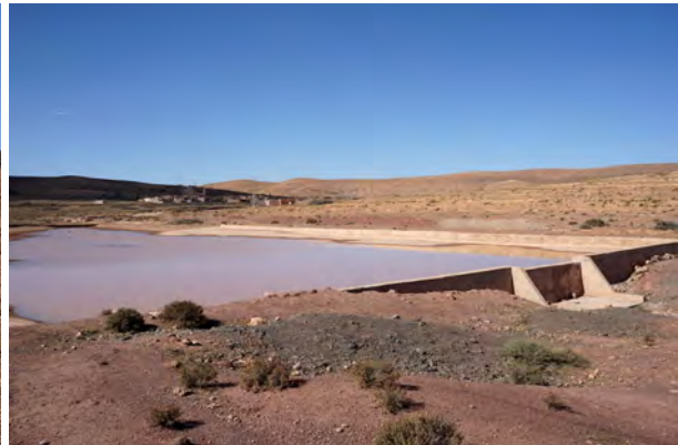
Fig. 71: Storage basin with a concrete dam retaining the water of a small episodic river north of area AN1b. Domain C, autumn 2015.
