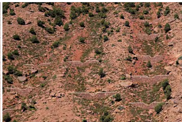
Fig. 47: Detail of fig. 46; erosion gullies that developed in the deforested part of a steep slope are stabilized with micro-dams. East of Aït Ouiksane, High Atlas Mountains, autumn 2015.
