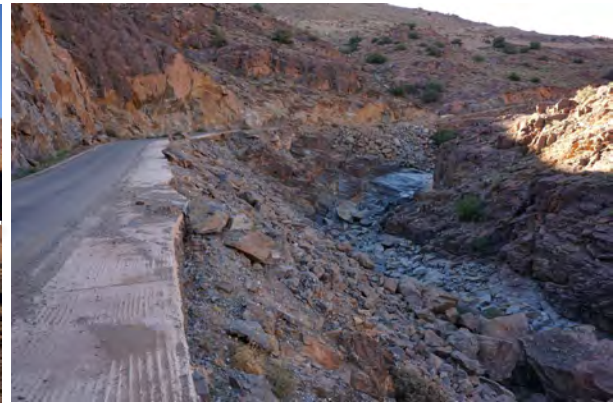
Fig. 120: Road through the lowermost Precambrian xl gneisses and migmatites at the beginning of the Aït Mansour gorge southwest of Tasserirt, view up the valley. The rocks in the dry riverbed are well polished, indicating periodical heavy floods. Domain A, area AS1a, autumn 2015.
