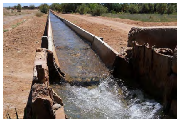
Fig. 98: Open channel for irrigation of large-scale plantations east of Ouarzazate. The water is pumped up from the artificial El Mansour Eddahbi lake near Ouarzazate. Spring 2011.
