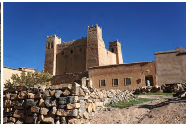
Fig. 127: Tighremt in Aït Moussa Wichou, built with unburnt clay bricks. Upper Dadès Valley, High Atlas Mountains, autumn 2015.
