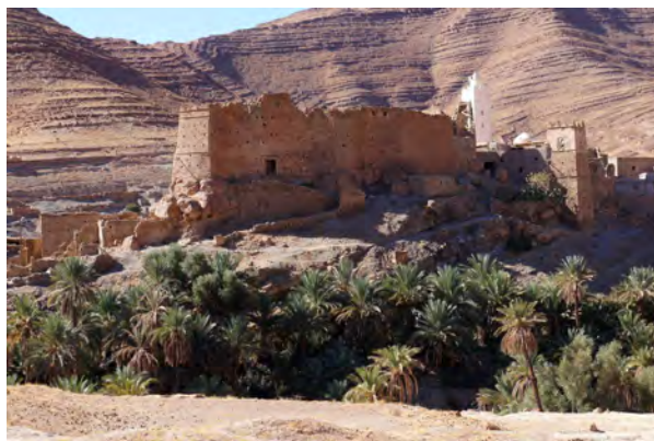
Fig. 196: Agadir (Berber storage castle) of Adghers N'Warfain that is about to disintegrate. Domain C, area AS4b, autumn 2015.
