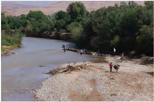
Fig. 85: Building of a dam with stones and sandbags to branch off an irrigation channel from Oued Dadès. Boumalne du Dadès, southern foothills of the High Atlas Mountains, spring 2015.
