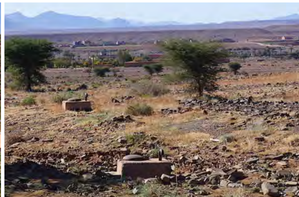
Fig. 139: Water pipe with shafts leading from cisterns on a hill down to the villages on the foot of the mountains. Alluvial plain south of Jebel Saghro (north of Nekob), autumn 2015.
