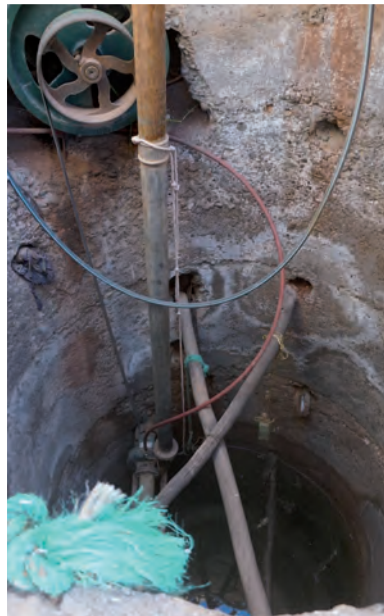
Former draw well recently equipped with a motor pump at Wa-Ou-Nsamt, High Atlas.
